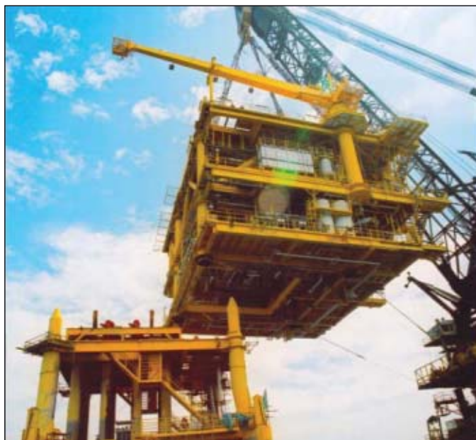
A crane barge lifted the 2,000-tonne deck on to the 24 slot-28 well, four-pile, 890-tonne jacket (Fig. 3).
