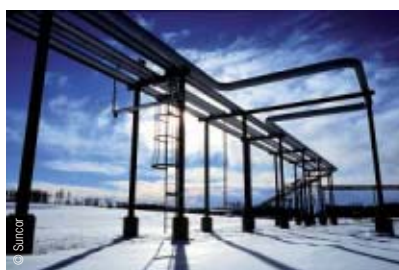
Natural gas plant, Alberta.
