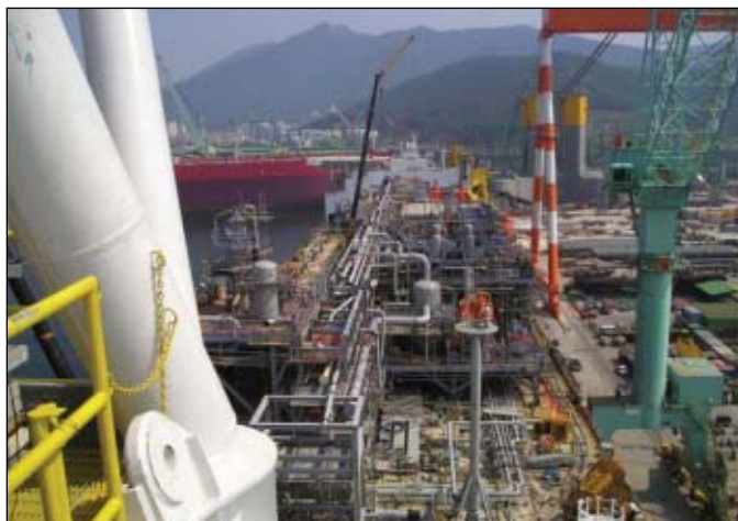
Module integration for the FPSO occurred at the SHI yard in Geoje, South Korea (Fig. 4).
